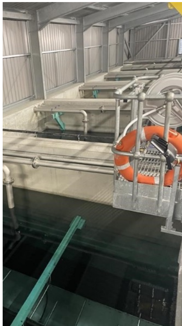
The new GAC (Granular Activated Carbon) filters plant at Tophill Low.
