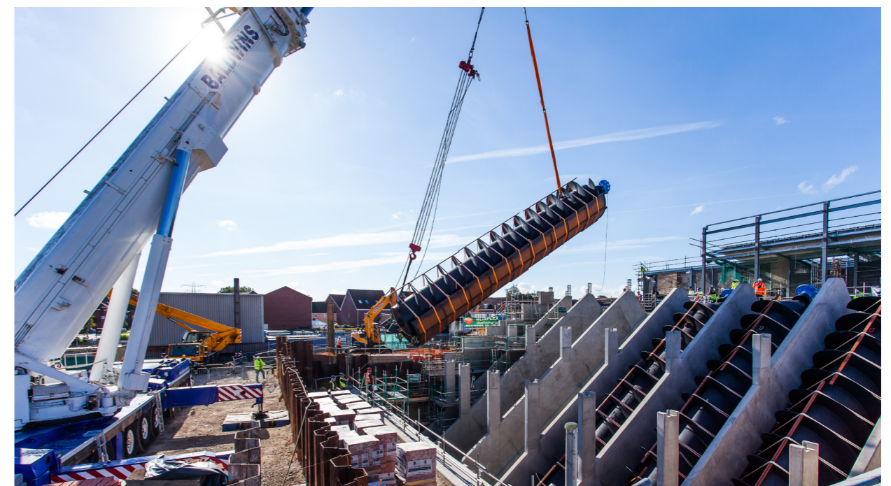
An indication of the scale of our infrastructure - installing huge new pumps at Bransholme Pumping Station in Hull
