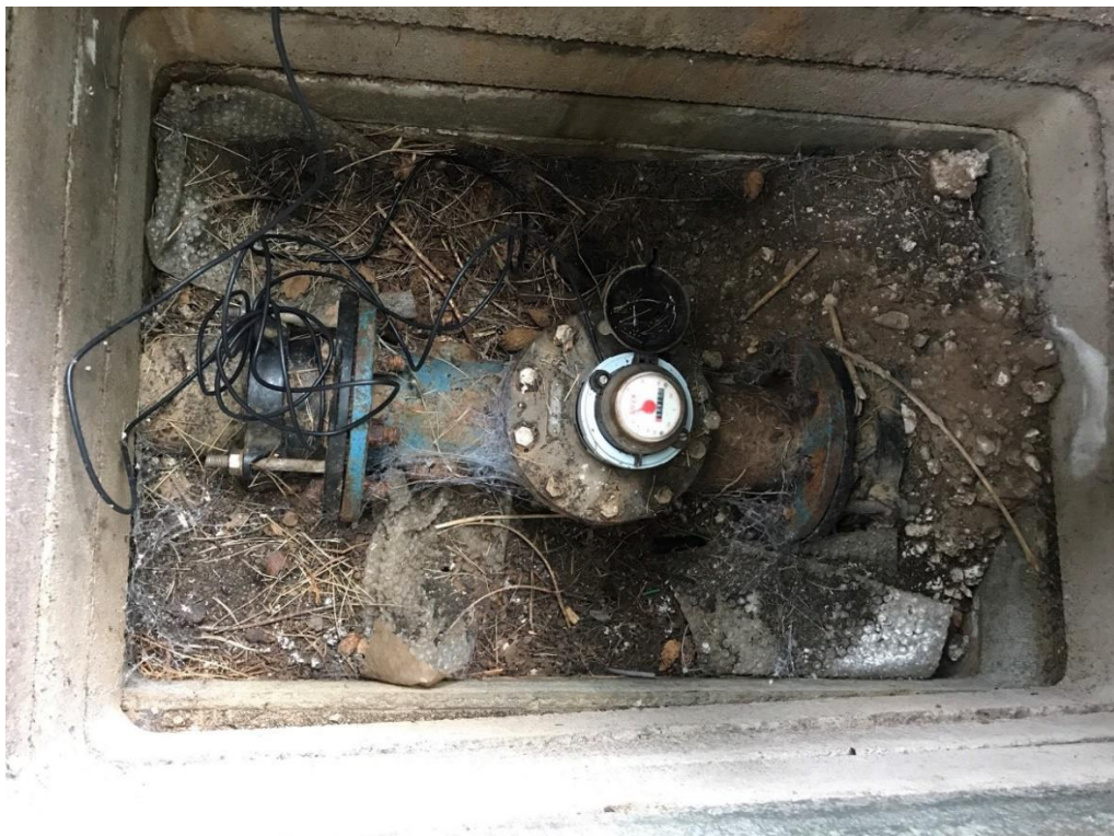
Figure 9: Green Hammerton inlet flow meter and bypass to be upsized to 200mm
