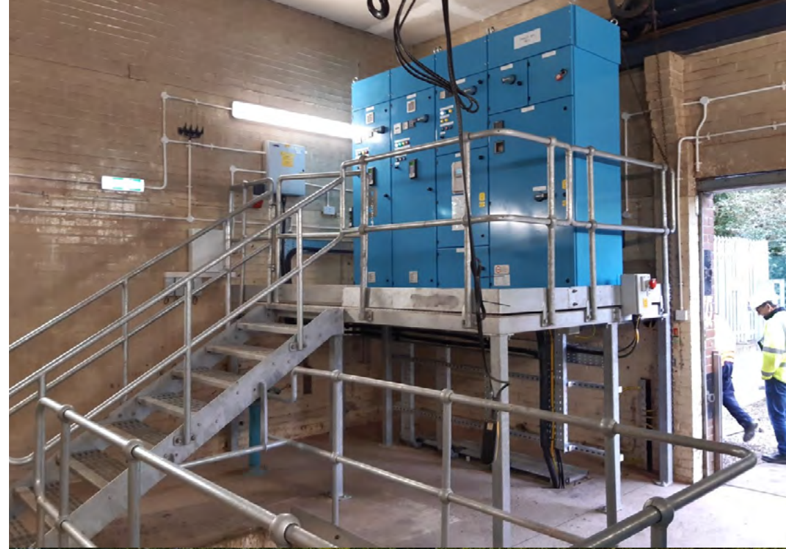
Examples of raised electrical control panels and kiosks to enhance flood resilience at wastewater sites
