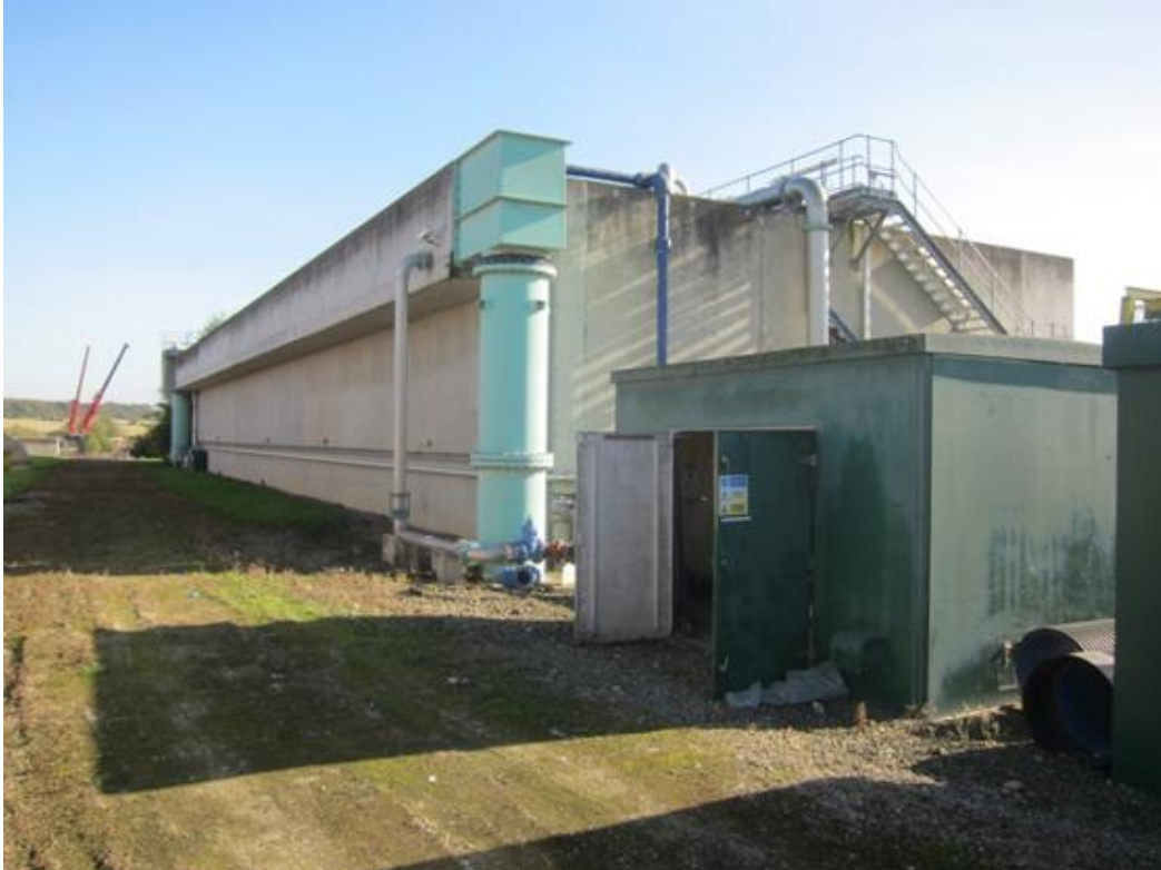
Figure 7 - The now redundant BAFF plant, showing HL works washwater pumping station (photo courtesy of B&V).
