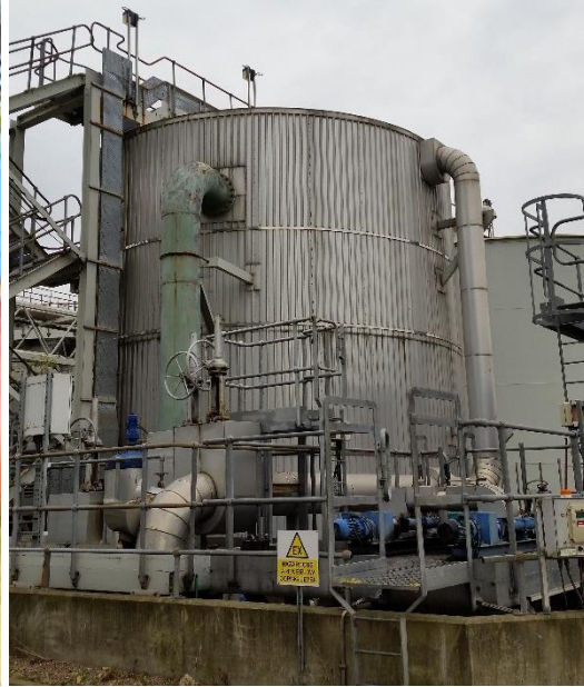
Figure 4 - The Treated Water Storage (FE) Tank installed near the incinerator
