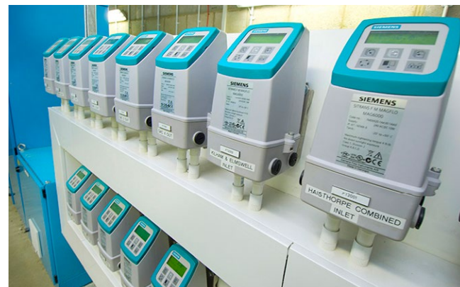
Haisthorpe Water Treatment Works
