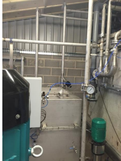
Figure 11: pumped outlet hotwell
