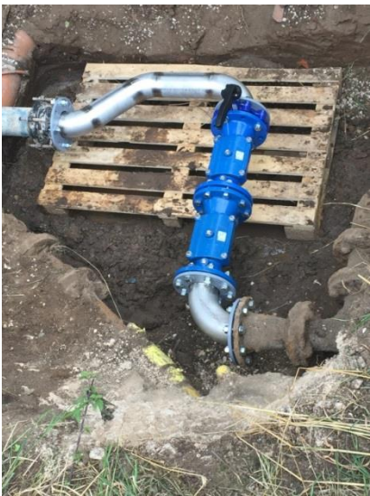
Figure 16: Double check valve installation
