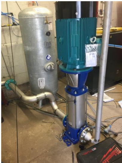
Figure 12: pumped outlet storage tank
