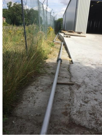
Figure 15: incoming mains after
