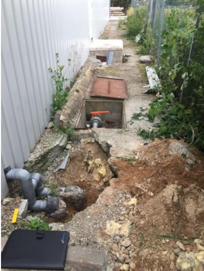
Figure 14: incoming mains before
