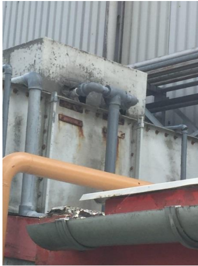
Figure 3: PPF storage tanks with incoming mains feed.
