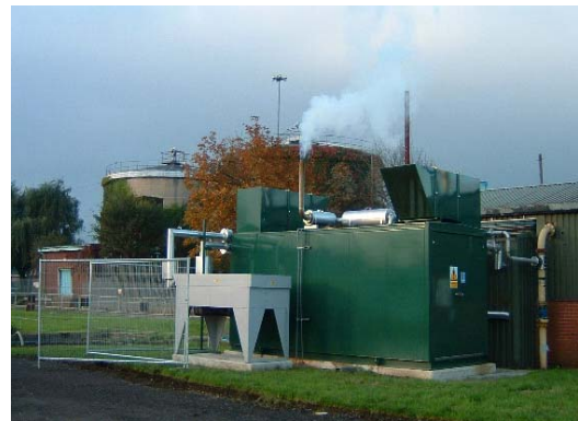
Figure 12: Mitchell Laithes CHP Plant
